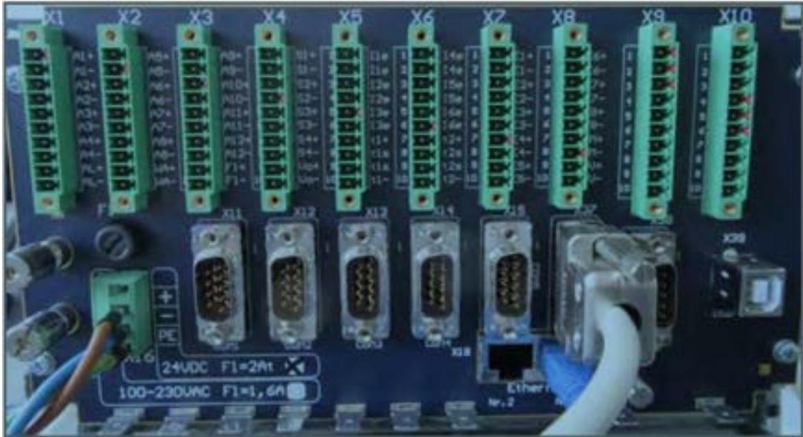
Fig. 8.18: Connection of the USM's Modbus interface to COM 6
